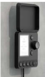
HMI control system on wall
